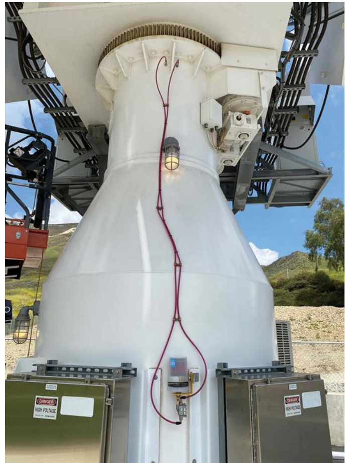
A 2-point MEMOLUB® Multi-Point System mounted for ground level access provides lubrication to the azimuth bearing.
