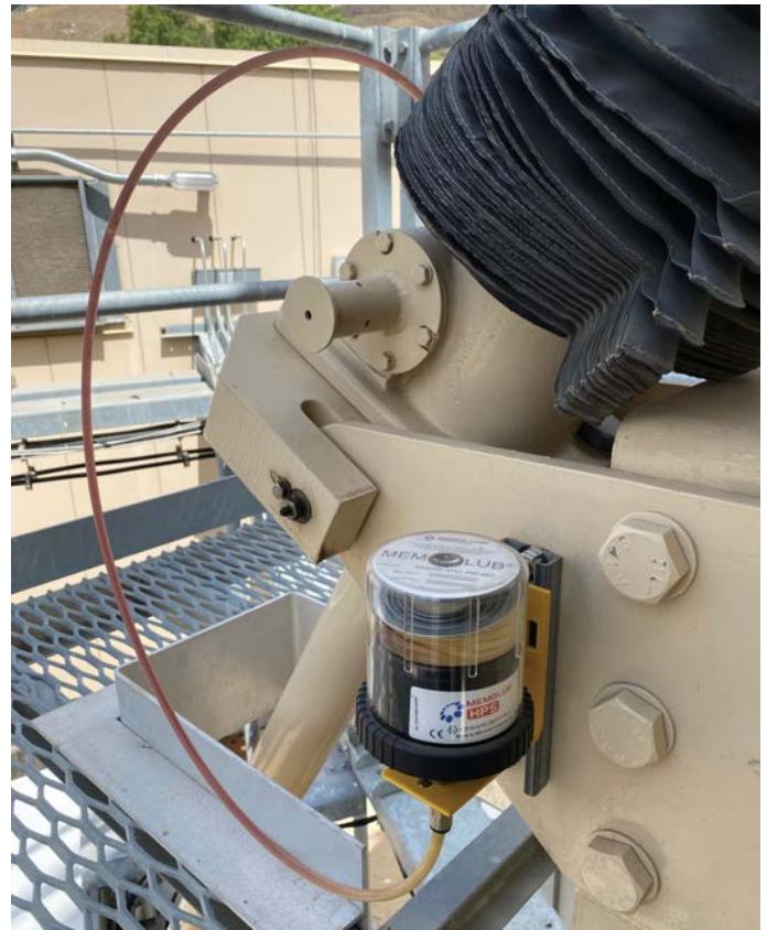
A remote-mounted MEMOLUB® single-point lubricator was used to service the elevation jackscrew housing on smaller antenna.
