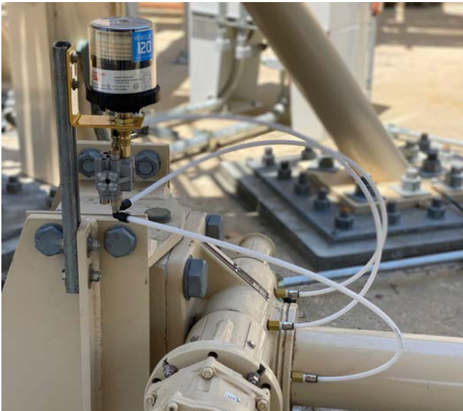
A remote-mounted 3-point MEMOLUB® Multi-Point System lubricates azimuth jackscrew housing on larger antenna.
